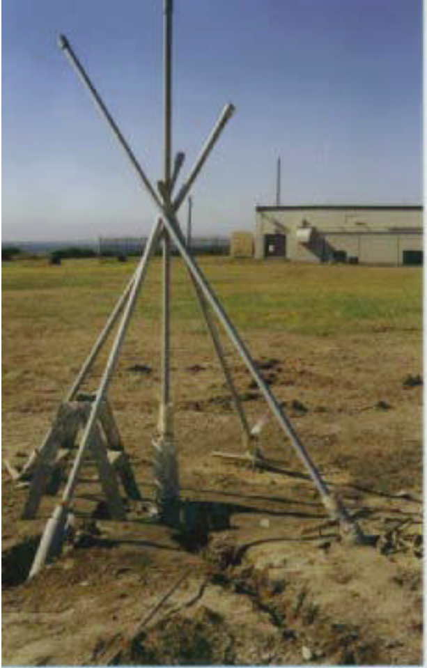
Figure 3. GPS site installation. Deeply anchored, drilled braced monument installed at Cape Blanco, Oregon. Each of five pipes drilled to approximately 12 meters depth, set in non-shrink grout, and isolated from soil and ground motions in the upper 4 meters by padded casing. The Pacific Northwest offers challenging conditions for stable site conditions. Much of the area is underlain by pervasively jointed volcanic rocks, poorly consolidated Tertiary strata, or other unstable lithologies. This monument was designed to provide stability under such conditions.
